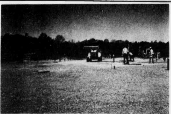
Now it looks like field of gravel, but plumbing and electrical work lie buried beneath. Soon cement will be poured for floor of Education Center.
