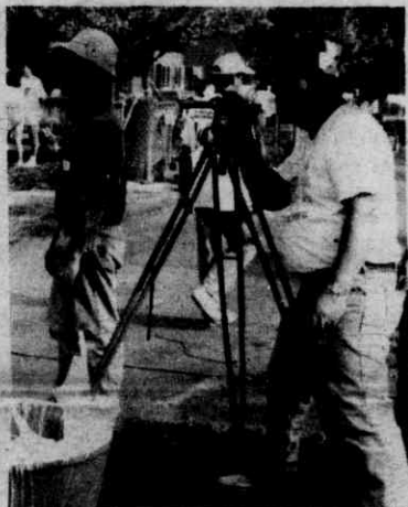
Herm Zeigler and Peter Hindel keep the playground installation on the level.
