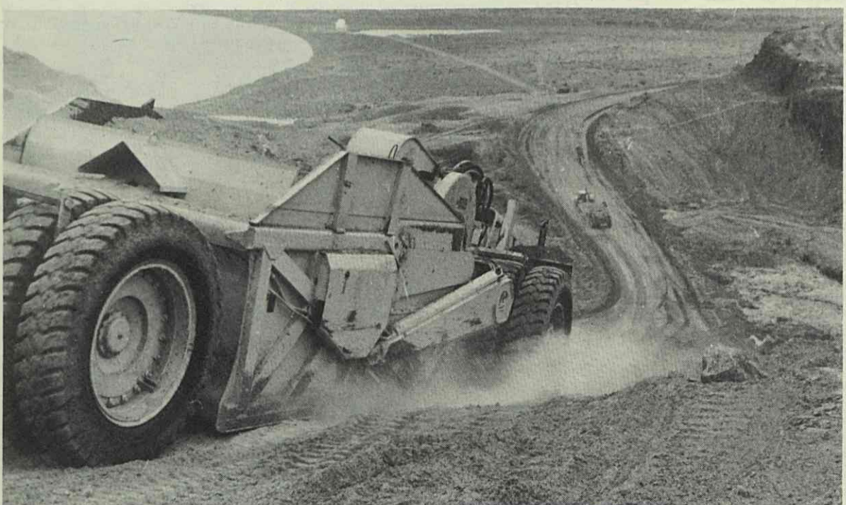
LARGEST SINGLE construction job ever serviced in the company's history was announced in 1962 when Firestone was designated tire supplier for the $345 million Mangla Dam project on the Jhelum River in West Pakistan, the first part of the huge Indus River development which will be more than seven times the size of the St. Lawrence Seaway development when completed.
