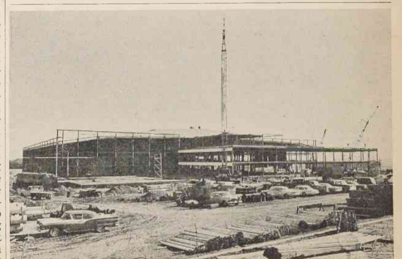
CLOSING IN for winter work on Piedmont's new home office and hangar facilities, the roof is nearly finished. Construction is right on schedule.
