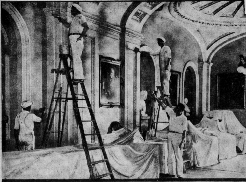
Painters are seen busily at work in the main corridor of the senate wing of the Capitol. A program of painting, redecorating, elevator installing, reconditioning of plumbing and general improvement such as has never been equalled since the British raid of 1814, has been under way. As a result it wouldn't be surprising if many congressmen fall to recognize the old place when—and if—they return.
