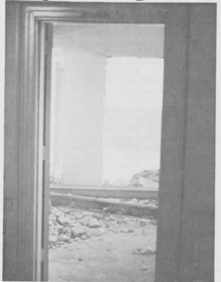
The Hardy Library is undergoing some drastic changes to become the new administration building.
