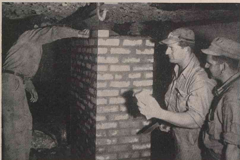
Above left: Bill Cline, Jess McCall and Paul Beddingfield of the Masonry Crew use air hammers to remove old-style beaters from refining room. Work assignments for the Masonry Crew often includes removal of old brick or concrete work, as well as putting in new work. Left: Joe Wright, Calvin Day and Calvin Frady put in new underpinning in reservoir pump house. Right: Replacing a wall in Electrochemical plant.
