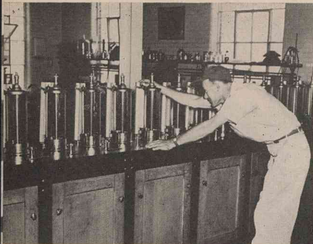
Harold Misenheimer is shown checking the water of number four filter bed at the sampling table. Water is on tap for instant testing on all stages of water treatment.
