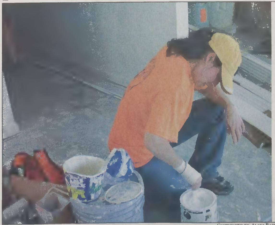
Junior Lydia Zimmer stirs paint while working on a house in New Orleans. Over spring break, 46 students traveled down to New Orleans to work on Katrina-damaged houses. The Key Center sponsored the event.
