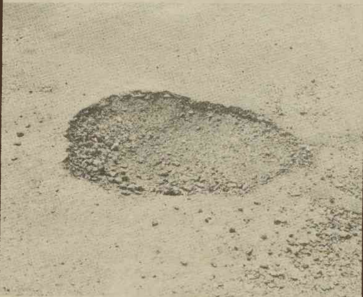
No, this isn't a crater found on some distant planet, it's an aged pothole located right here at Brevard College--and it's a roadway killer! Those BC motorists lucky enough to dodge this one (located on the drive below the music building en route to the gym and SU) risk damaging their autos on several others that lurk in our streets. Maintenance better do something soon before students begin to lose not only front-end axials, but whole cars!
