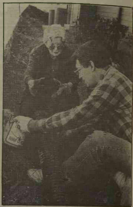
During the Faculty Work-Play Day held on Oct. 27, Preston Woodruff helps repair a drain pipe at the Frances Warde Health Service outside Rosman. He is helped by one of the nuns, Jacquie Dewar, who works there, (Clarion photo by Jock Lauterer)
