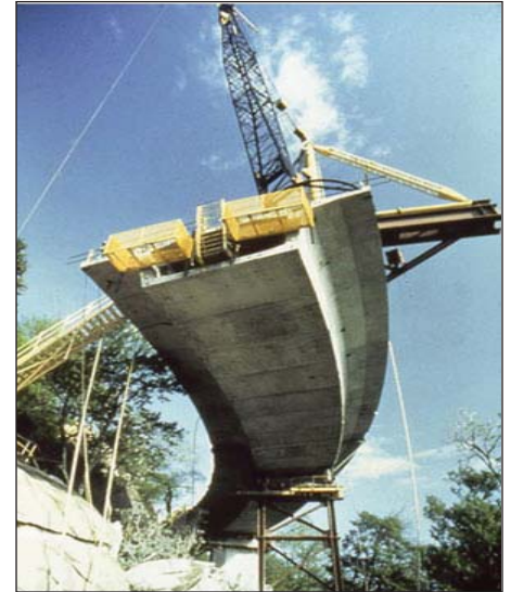
The Linn Cove Viaduct, finalized in 1987, opened the full 469 miles of the Blue Ridge Parkway, allowing travelers to drive from Shenandoah National Park all the way to the Great Smokey Mountains National Park.
