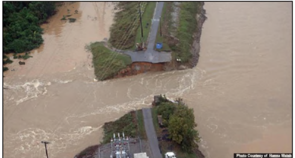
A road crumbles as a result from the floodwaters in Columbia, SC.
