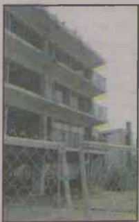
This dilapidated hotel is one of several decrepit areas still visible downtown.
