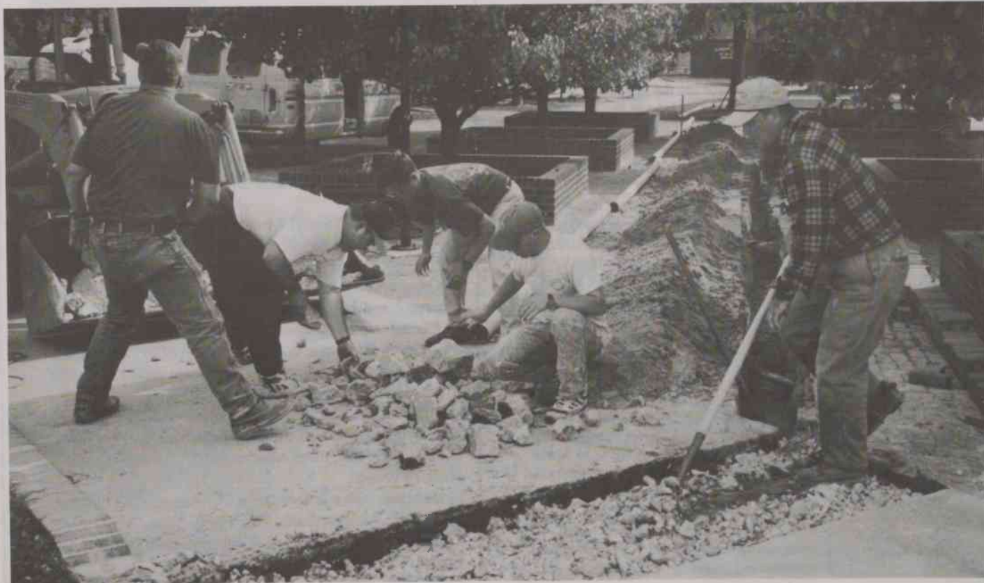
Members of the Chowan maintenance department, under the direction of Johnny Brock, director of physical plant, prepare the trenches to carry fiber optic cable under walkways and into the campus buildings.
