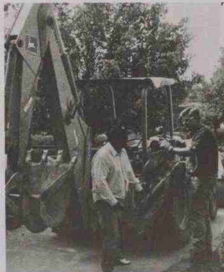
Johnny Brock gives directions to the backhoe operator as to where to begin digging a new trench for the fiber optic cable.
