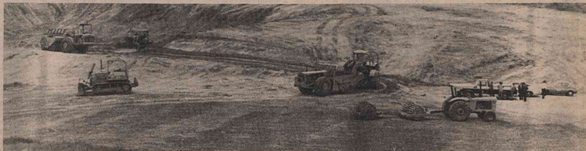
PREPARING THE SITE—Like so many dinosaurs from ages past, over the last several weeks bulldozers and grading pans have been making their stately and earth shaking progress around the basin which will one day hold Duke North Hospital. While it looks like they're just driving around in circles to the average sidewalk superintendent, according to one of the drivers, there is method to their
