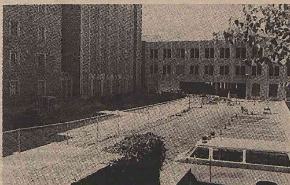
MAKING WAY FOR THE PRT —About half of the emergency driveway has been fenced off for construction of the lobby for the Duke South terminal of the transportation system which will link the present hospital with Duke Hospital North. (Photo by John Becton)
