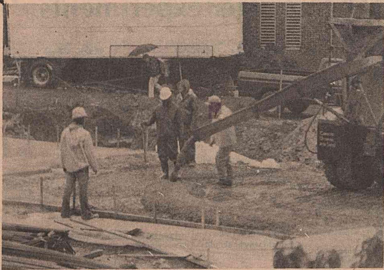
NEITHER RAIN, NOR... — Workmen were undisturbed by the rain late last week as they poured concrete for the PRT (Personal Rapid Transit) track, between the Bell and Mudd Buildings. The PRT will link Duke Hospital North and Duke Hospital South, and people going from one to the other will be undisturbed by rain or other inclement weather which might be around at the time. (Photo by John Becton)
