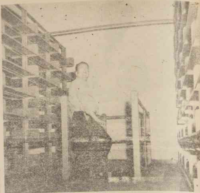
A view of the new second-level book stacks in the Elon College library is shown above in a photograph taken when the installation of the new shelves was completed recently. The installation was under the supervision of Joseph Acquaro, of Cincinnati, Ohio, who is a representative of the Globe-Wernicke Co., also of Cincinnati. The new stacks double the book capacity of the Elon stack room and serve to relieve the badly crowded condition that had existed on the shelves for some time.
