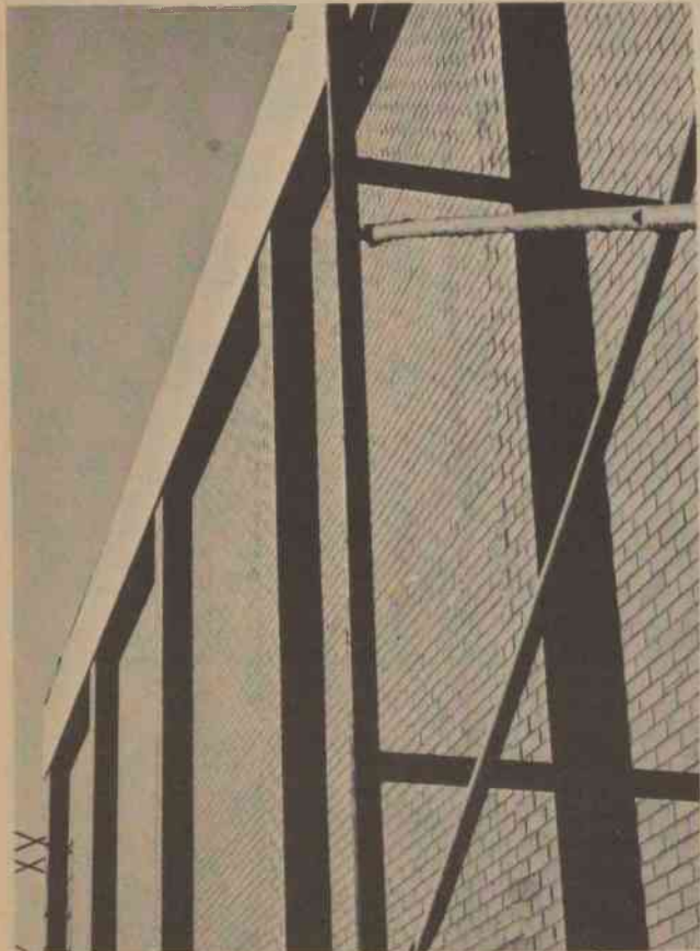
Photographer Robert Wicker found a bit of modern art in the construction of the new physical education facility. The building is scheduled for completion in the summer.
