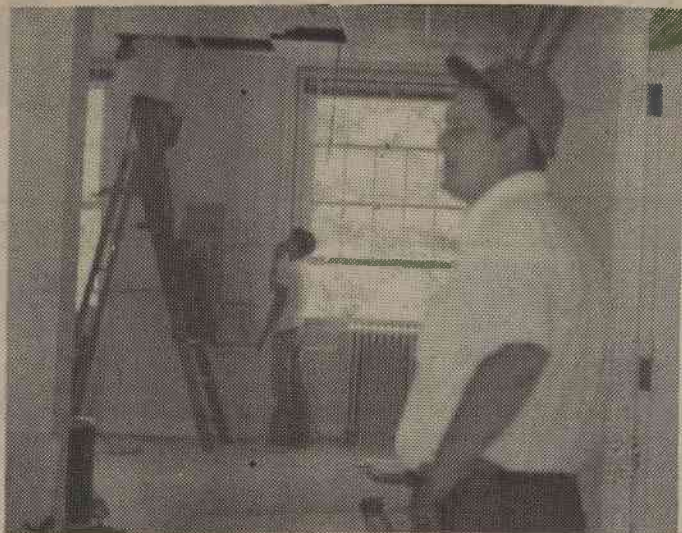
Physical plant director L. B. McCauley watching renovation of Mooney progress. (Photo by Lance Latane)
