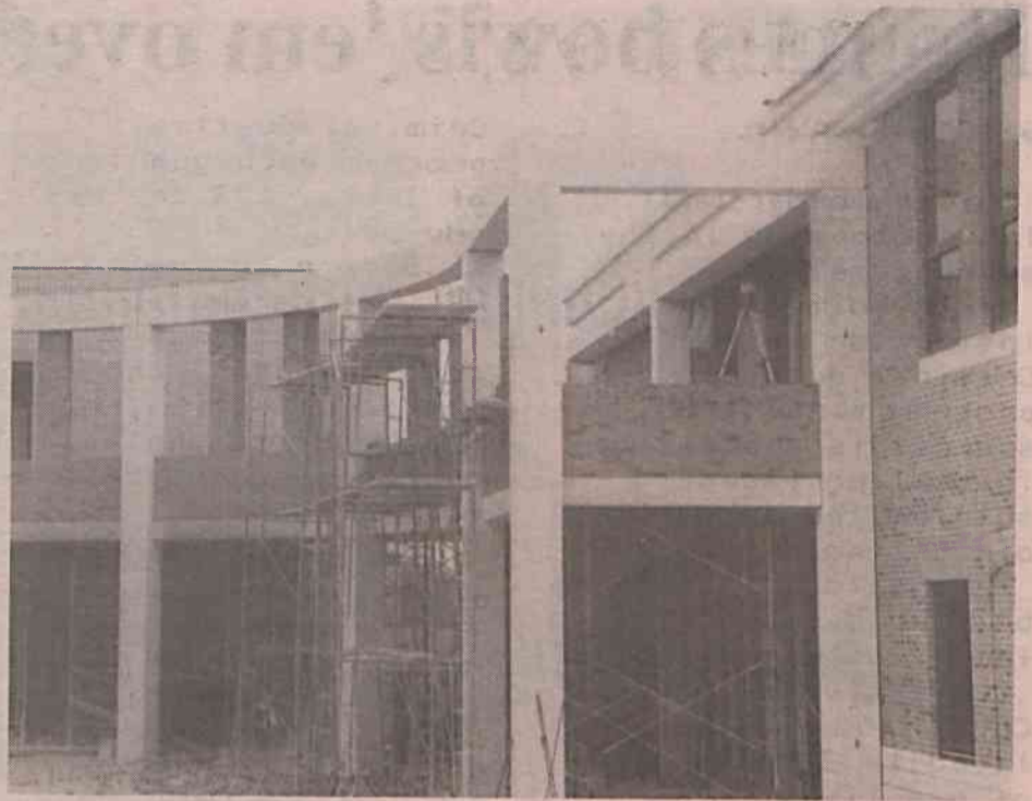
The walkway that adjoins the Arts and Mathematics Building with the Mechanical and Social Science Building in early stages of construction. PHOTO: Todd Howe
