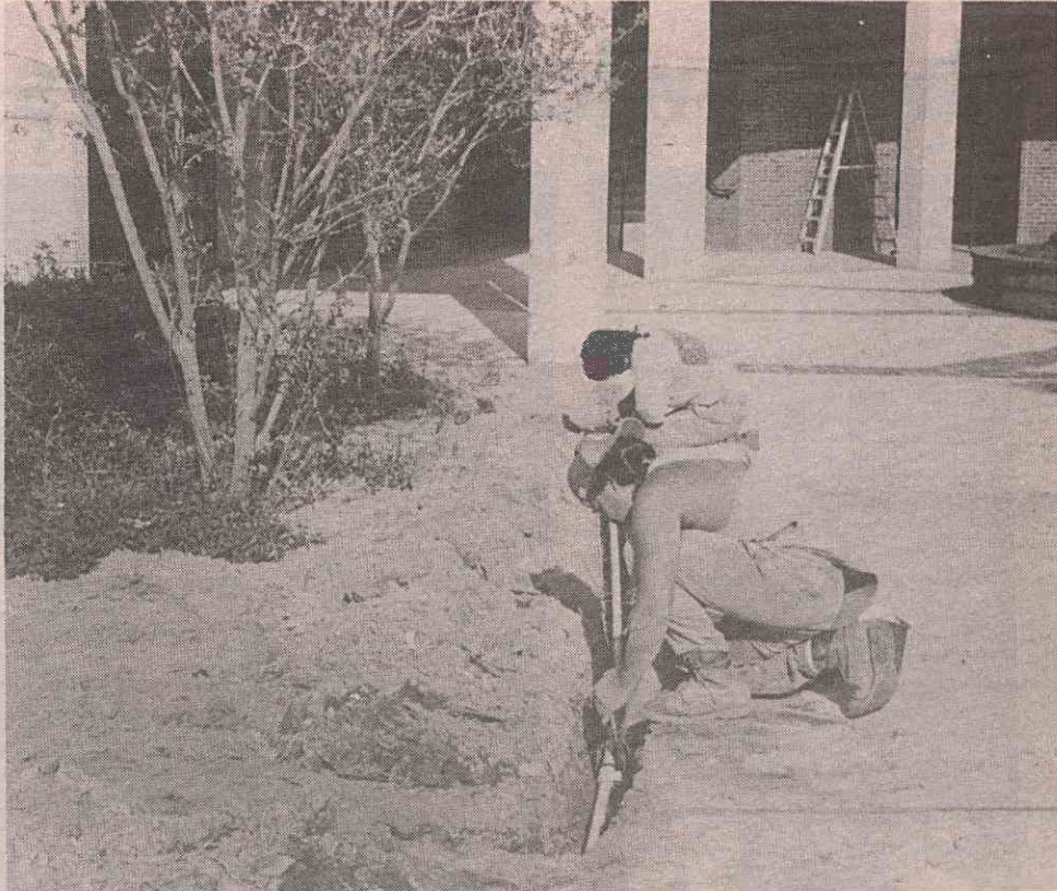
Larry Martinez, front, and Bicno Francisco, workers with Landscape Design, install sprinklers outside the A&A building.
