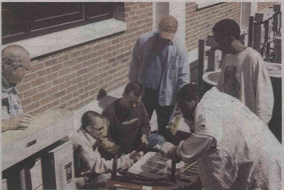
Heating and air conditioning students and their instructor repair a unit (l to r): Robert Garner, Michael Smith, James Cartwright, Michael Bingenheimer, instructor J.E. Bass, and Charles Lucas.
