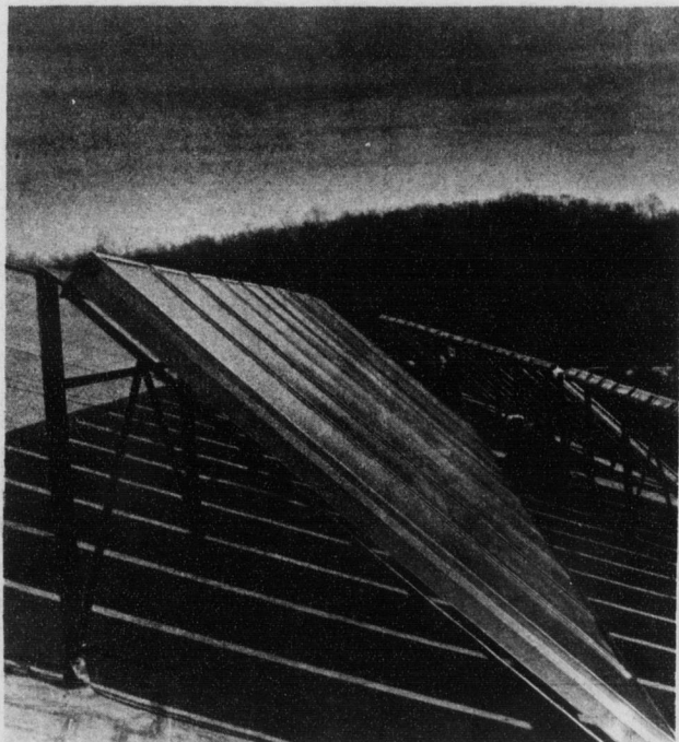
Solar panels atop alumni gym
