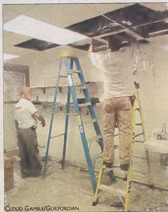
George Hendrix (left), working for Triad Sheet Metal, and Jay Fletcher, with Frank L. Blum Construction, work in the pizzeria kitchen.
