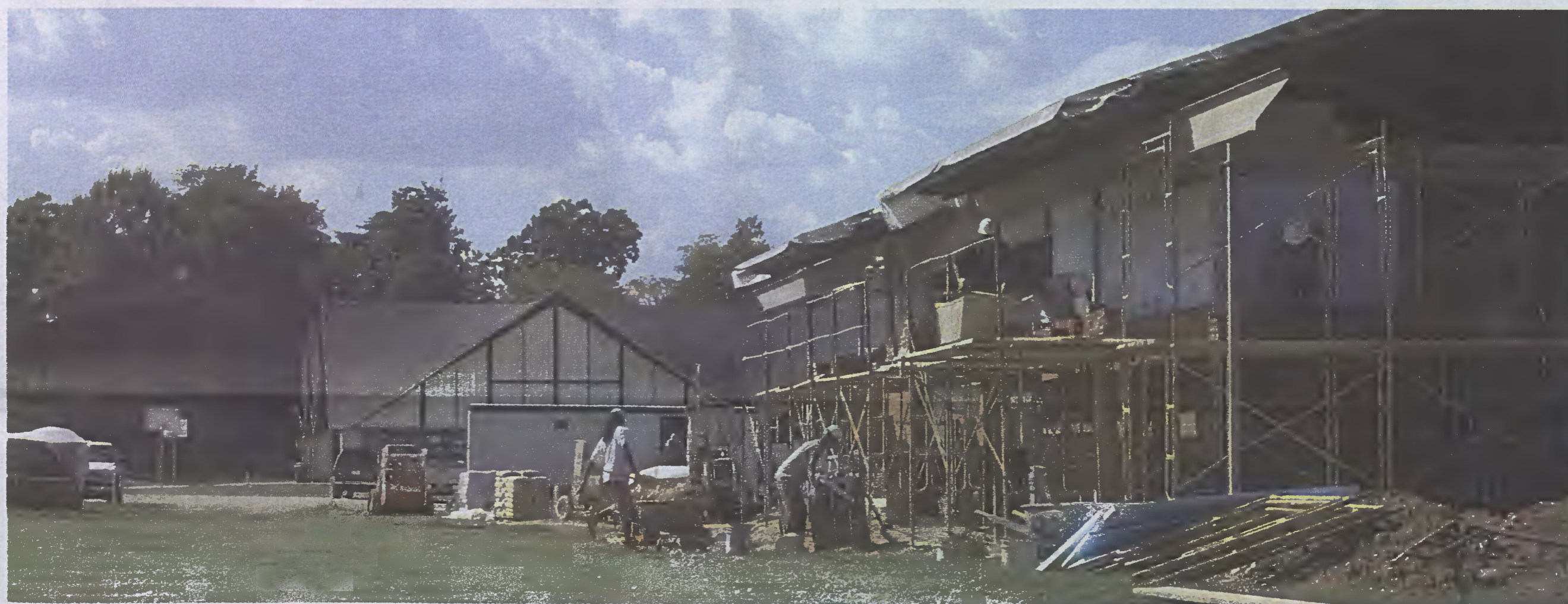
The Jack Jensen Golf Center is currently under construction behind the Ragan-Brown Field House. Herb Appenzeller donated six months' royalties from one of his books to help fund the facility.
