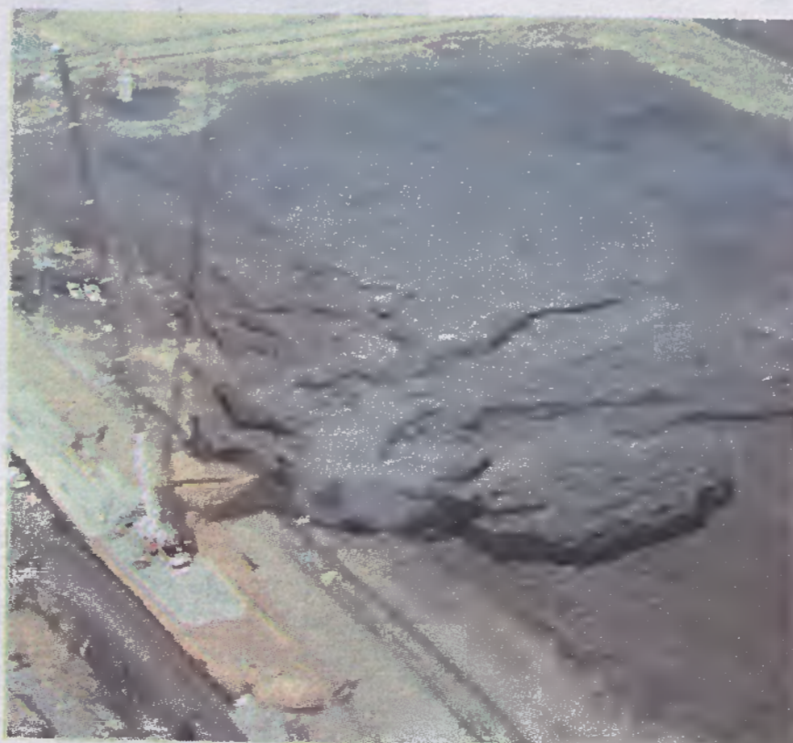
A broken storm drain under a storage pond in Eden owned by Duke Energy caused the third largest coal ash spill in U.S. history.
