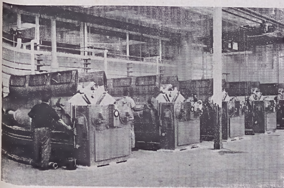
Recently-purchased jig dyeing machines are shown in the new jig dyeing department at the Blanket Finishing Mill. Jigs from the old department will be moved to this area soon. The operators shown are Matt Roberts, front; Ralph Lindsay, middle; and Tommy Hairston.
