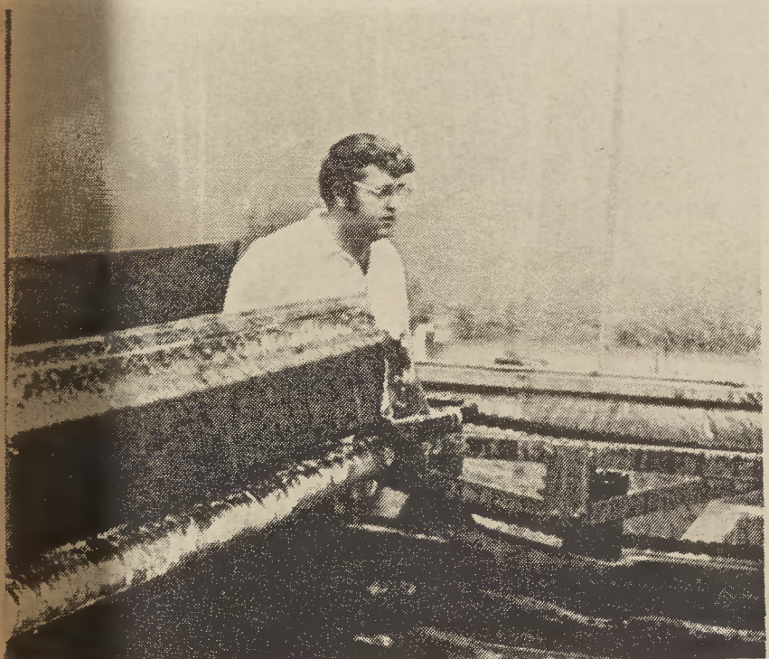
John Everette is head water plant operator.
