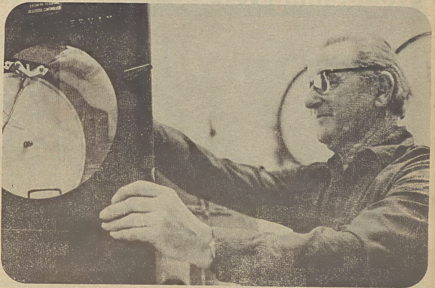
Payton Jeffries, first shift, changes pre-chlorinator charts which show a record of how many pounds of chlorine are added to raw water each day.
