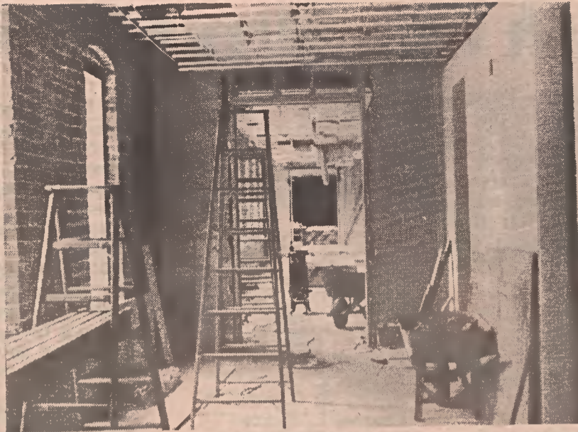
WHILE WORK WAS in progress, all ceilings and the entire interior was torn out except for weight supporting walls.
