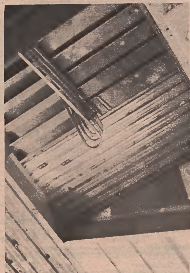
ALL THE HAZARDOUS wooden stairs were replaced by concrete and metal, fire-proof stairs like these.
