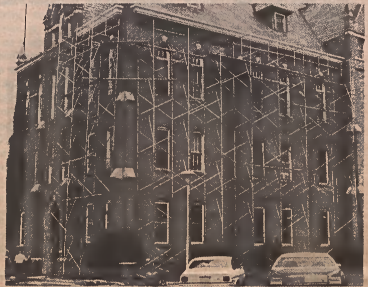
St. Leo's Hall is receiving a face lift. Minor renovations include roof repair, interior wall painting, resurfacing of floors, and renovation of rest rooms. Your contributions at work!
