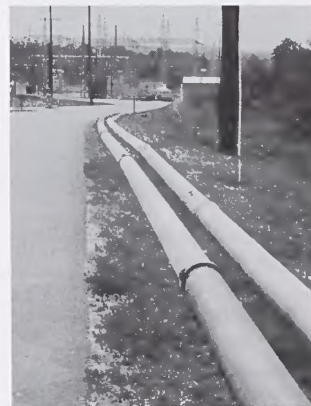
Pipe lines parallel entrance to plant.
