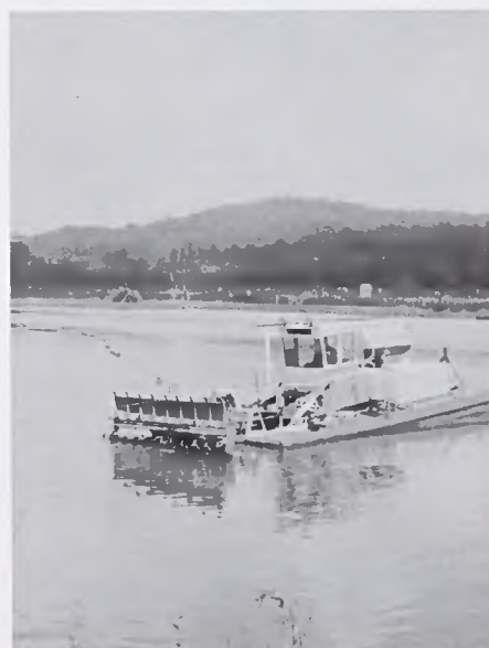
Barge in settling pond pulls dredge out of water to show how it will work.
