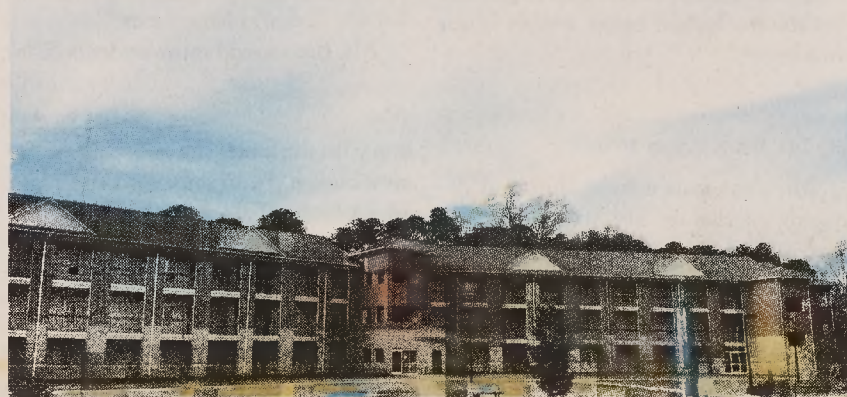
The Falk Crest A and B dormitories have structural problems on the first floor.
