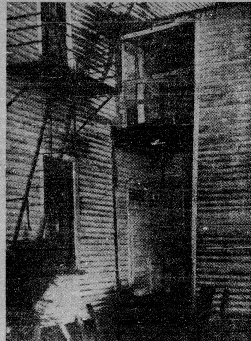
400 STUDENTS' PROTEST SCHOOL CONDITION—Another view of Redstone Academy, above, reveals a fire escape and a sagging door and bridge between the main building and an annex where toilet facilities for girls are located, the rotting weather boarding and a sagging door. Students entered the third day of their strike in protest against these conditions which are termed "safe" by school authorities. (News and Observer photo by Stephens)
