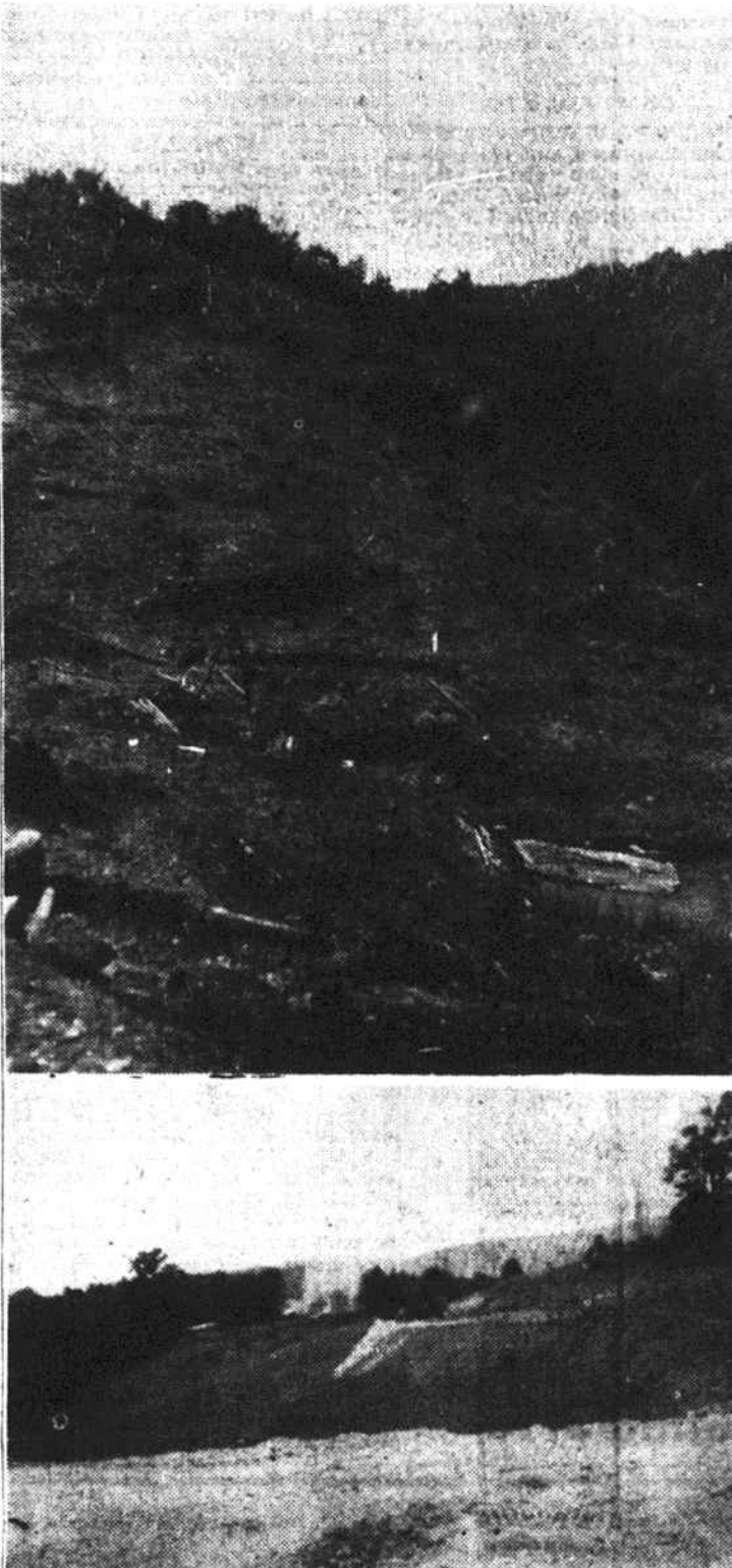
Above is shown the site where Julian Price of Greensboro, is building a lake, near Blowing Rock, on Boone's Fork. Bottom view is of the approach to the development from the John's River road.
