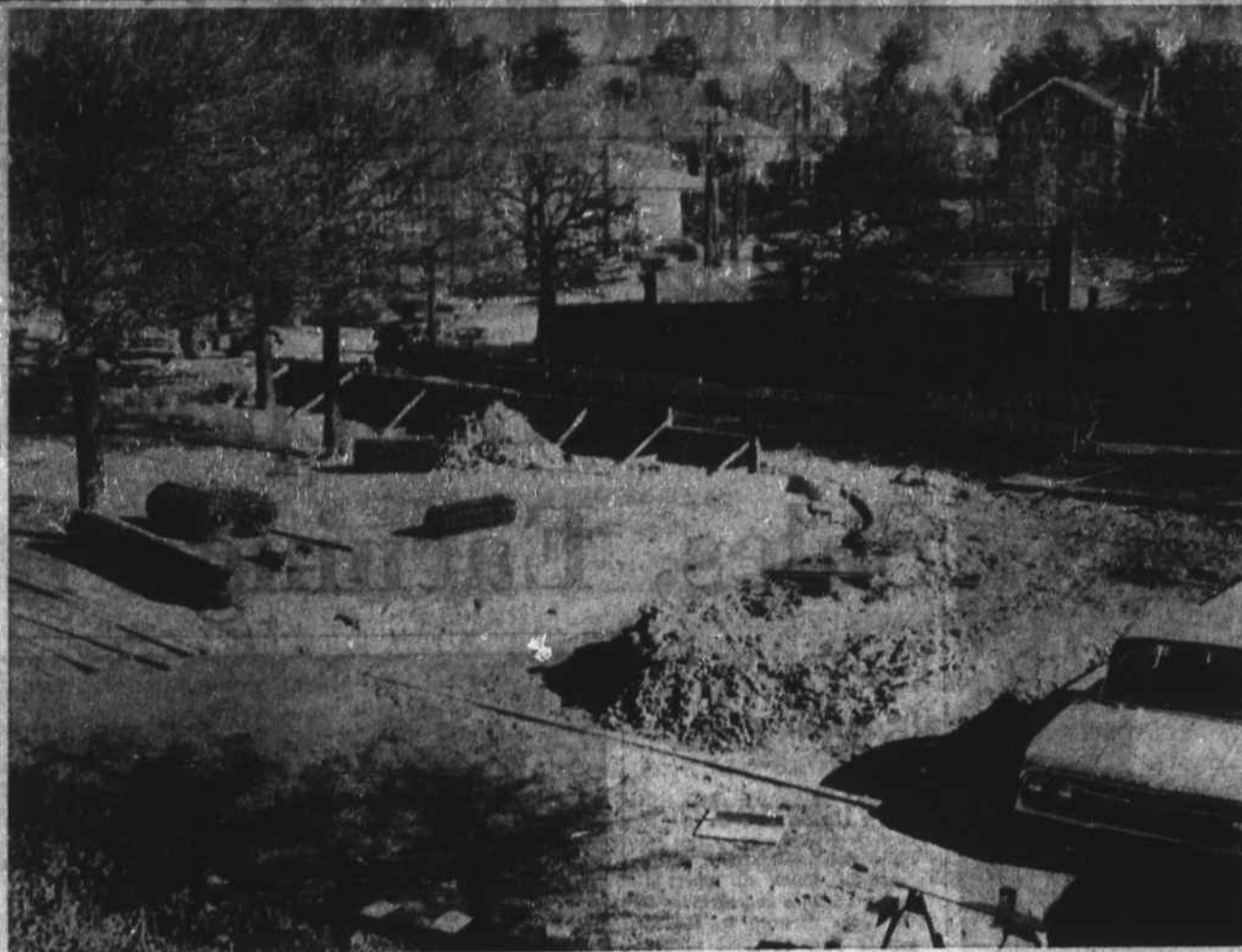
IMPROVEMENT.—The cold weather this week halted progress on the back entrance to the Boone Post Office. The driveway, entered from Queen Street, is expected to aid in getting the highway post-offices into the parking lot of the local post office, Ralph Greene, acting postmaster said. The buses will be able to drive in forward
