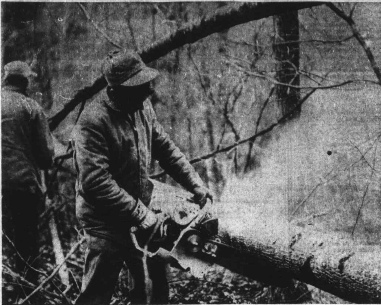
ON STADIUM SITE.—Workmen clear away trees and underbrush on the site of Appalachian State Teachers College's new football field. The stadium, when completed, will replace the one now being used, beside the men's old gym.—ASTC News Bureau photo.
