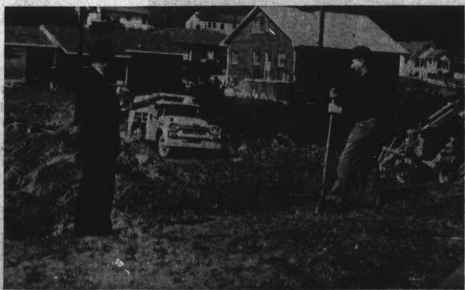
FUTURE APARTMENTS.—An eleven-unit apartment building is under construction on the Blowing Rock Road near the campus of Appalachian State Teachers College. Being built by Estel G. Wagner and Cecil Miller, the structure is expected to be completed
