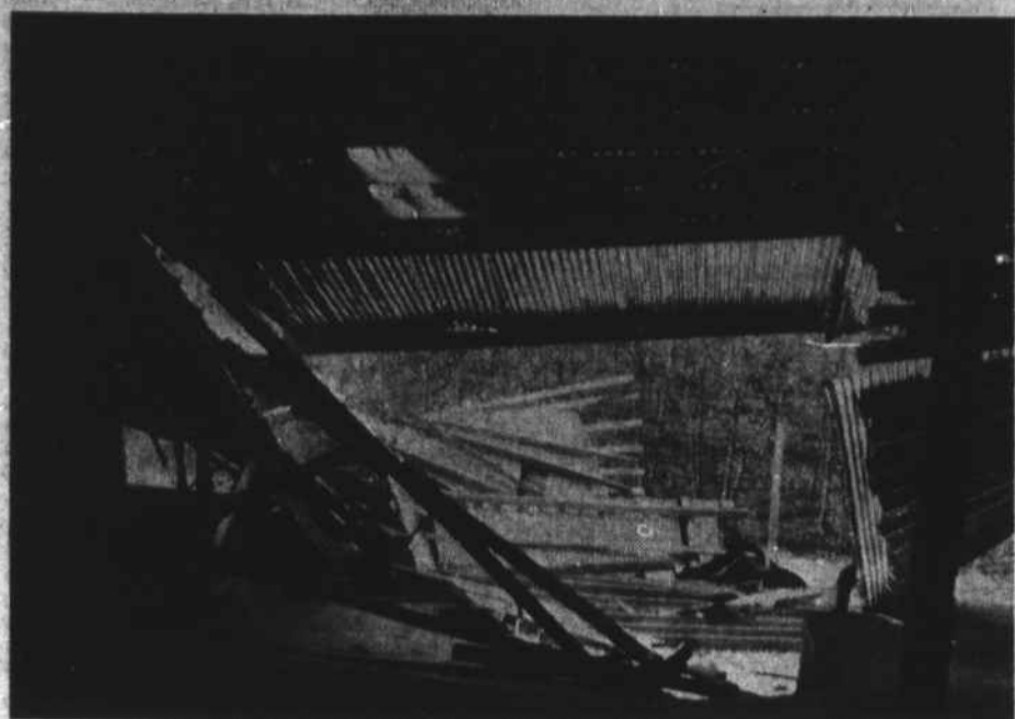
BETWEEN $3,000-$5,000 DAMAGE. —Strong winds caught a north corner of the recently constructed Big Burley Warehouse on N. C. 105 about two miles west of Boone last week, tearing back a portion of the tin roof and causing a section of
