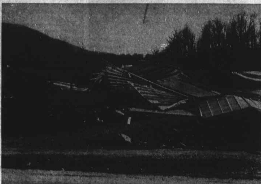
one wall to collapse (left photo.) The twister pushed the supporting beams away and forced part of the huge roof to the warehouse floor (right photo). S. C. Eggers, local personnel official for the warehouse, stated that insurance ad-
