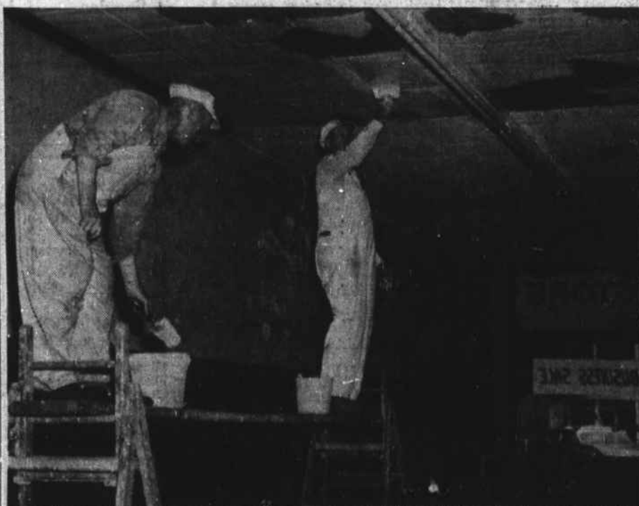
Painters Ralph Wilson (left) and Roy Ruffy are shown as, several weeks ago, they began their part in transforming the Boone Tire and Bargain Store building into the new Boone Variety Store.
