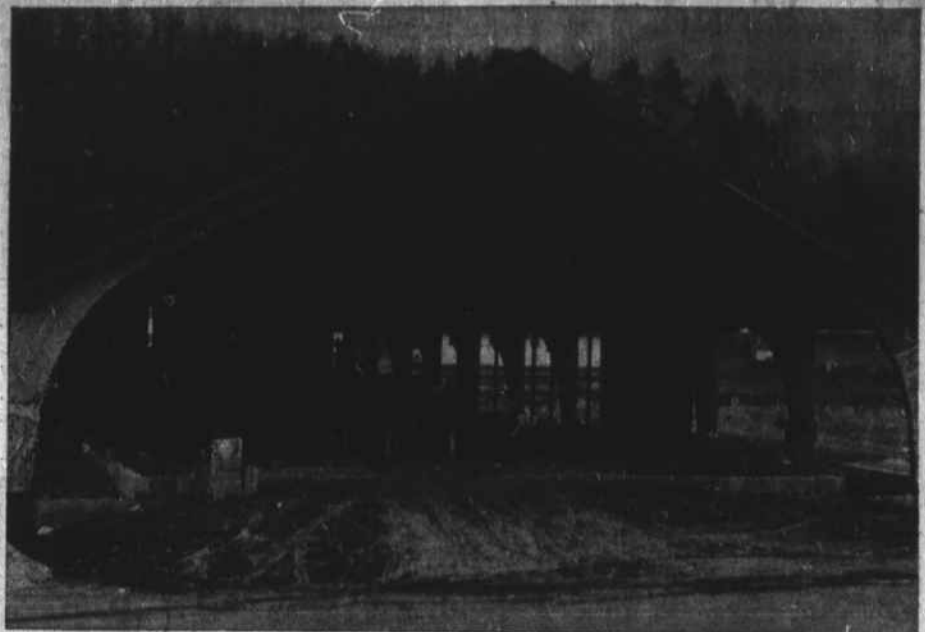
The main part of the new addition now under construction at Greenway Baptist Church, with part of the new educational section of the church in the background at left.
