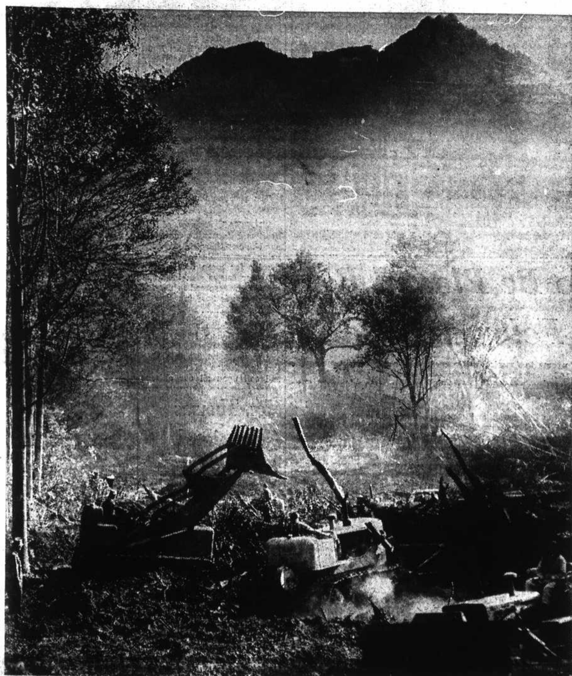
COMPLETING CLEARING ON NEW COURSE—Smoke from brush heaps and early morning mist rise from the Linville River Valley toward the towering peaks of 6,000-foot Grandfather Mountain as bulldozers put the finishing touches on clearing
