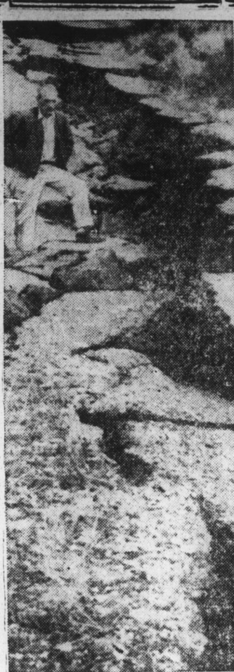
CENTER LINE — A forestry worker stands near a crack in the road at West Yellowstone, Mont., following the earthquake that struck the area.
