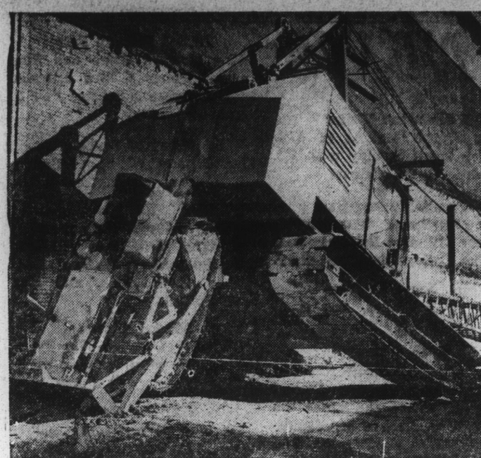
BIG BULLY-DOZER —What looks like a fight between two mechanical monsters actually is the result of a freak accident. The small bulldozer was being used to help weight down the larger as it tried to lift its block-long boom. The boom was too heavy, and the weight lifted the cab off the ground, with the little one trailing behind in Dallas.
