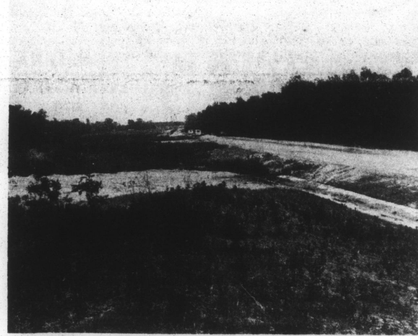
CROSSING PEMBROKE CREEK —Work has begun on the bridge over Pembroke Creek which had delayed completion of the U. S. 17 by-pass. This picture was taken looking east toward the creek.
