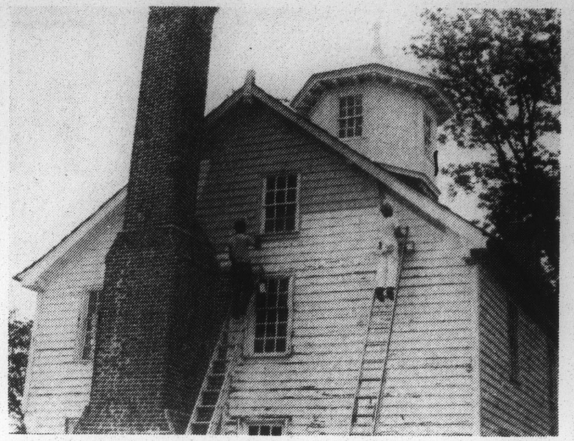
FACE LIFT — Local painters are giving the historic Cupola House fresh coats of paint for a new appearance. Work began this week to paint the landmark its original color, beige. The project is the result of work by restoration specialists with the Division of Archives and History.
