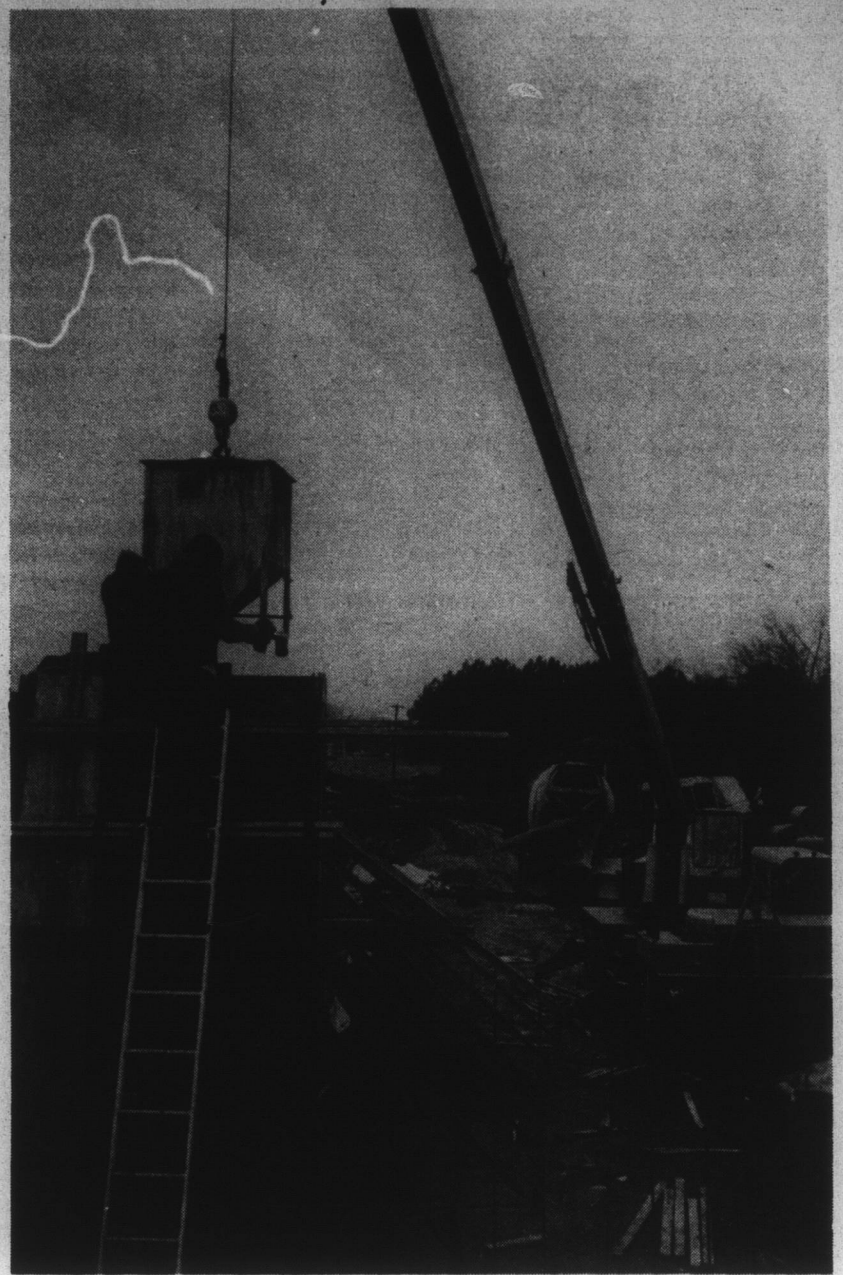
NEW CONSTRUCTION — Workmen are shown here pouring concrete at the site of a new solid waste transfer station for the Town of Edenton. The station, the first of its kind in this area, is being developed near the Municipal Garage, between North Broad and North Granville streets. (Staff Photo by Luke Amburn.)
