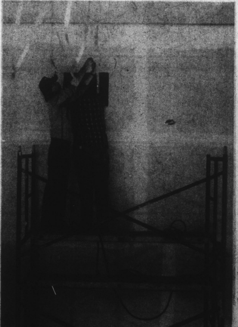
PROJECTOR EYE VIEW —Pictured here are workmen as they are preparing the new Taylor Twin Cinema for its spring opening. They are installing ductwork for the new heating and cooling system and are being viewed from the projector's angle.
